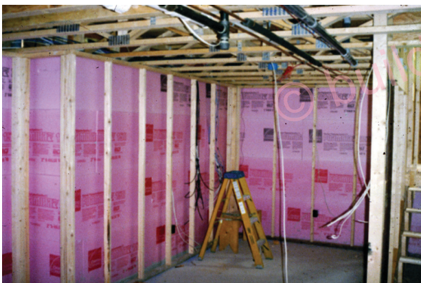
Figure 31 Rigid insulation can be installed in basements above concrete floor slabs and coupled with a floating floor
