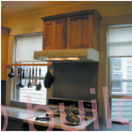
Kitchen exhaust hood
