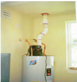
Power vented hot water heater
