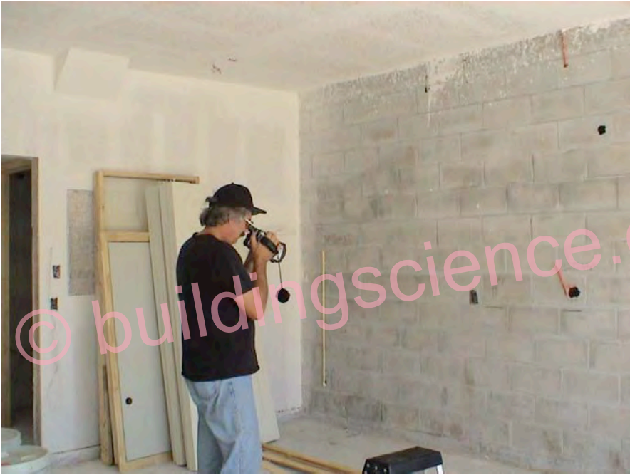
Photograph 44: Infrared Camera Leak Detection
