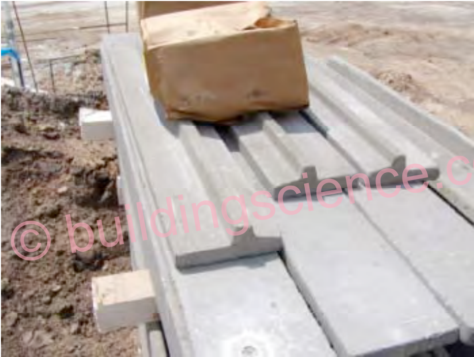
Photograph 27: Precast Sill With Illogical Attachment Rib
