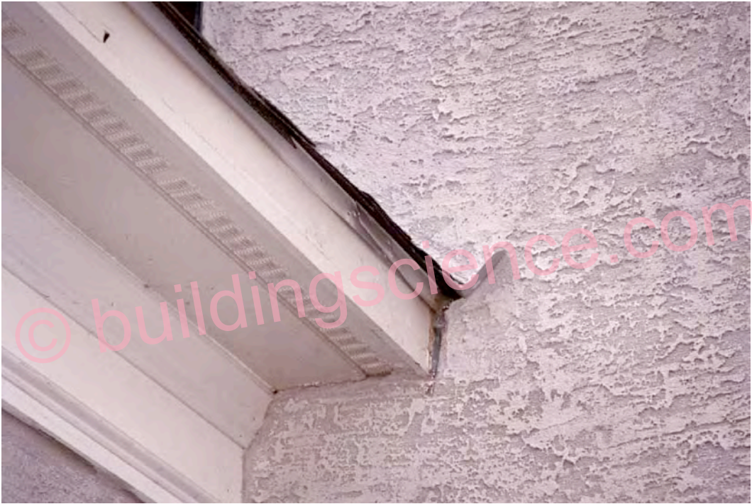
Photograph 39: Kick Out Flashing
