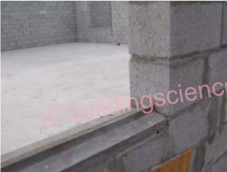
Photograph 28: Precast Sill That Channels Window Leakage Inward
