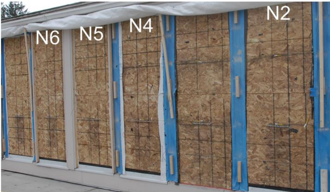
Figure 36 : Exterior OSB sheathing on the North orientation immediately following deconstruction (photo taken from the opposite direction of Figure 35)
