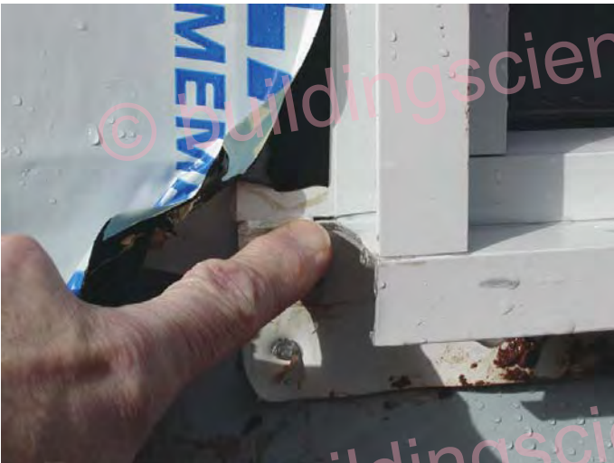
Figure 22: Cracked nailing flange at corner connection
