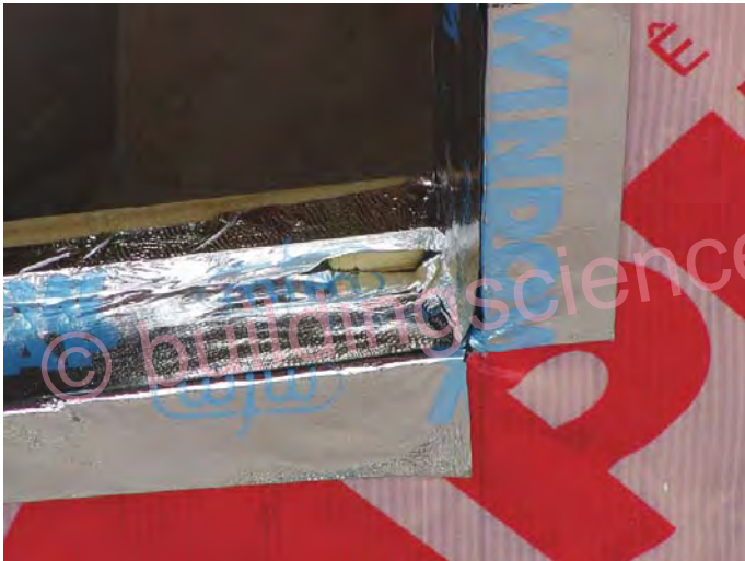
Figure 27: Torn membrane pan flashing
