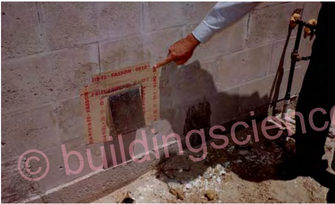
Figure 16: Membrane flashed exhaust vent
