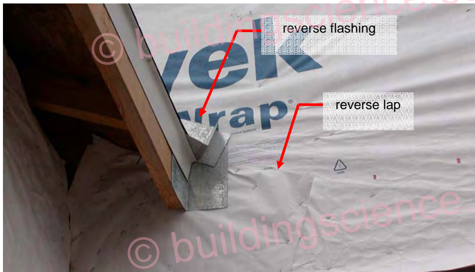
Figure 2: Improper installation of drainage plane materials
