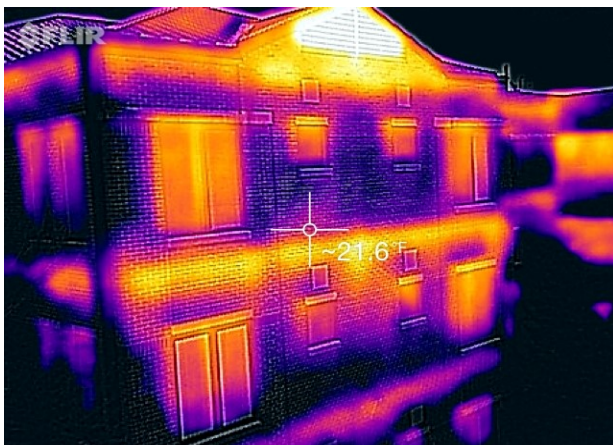
Figure 2: Gross air leakage visible on exterior building enclosure/shell
