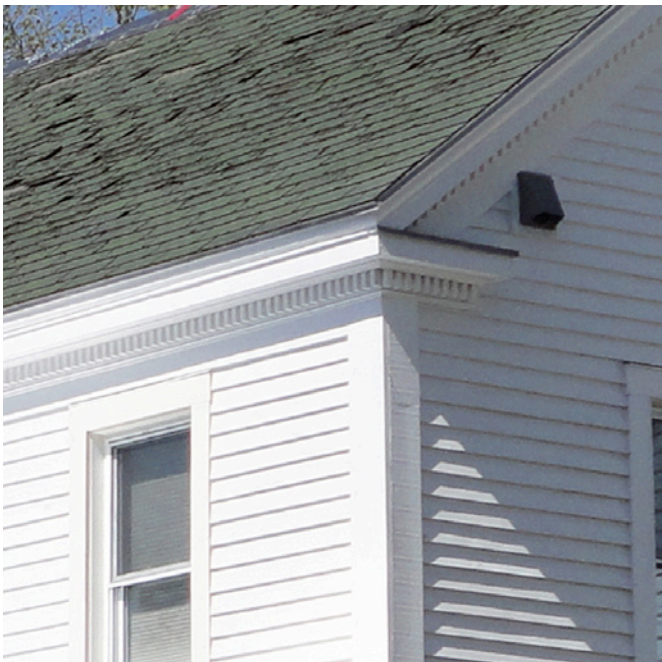
Photograph 5: Time To Replace Shingles —Note the condition of the shingles. Yes, it was time to replace them. Now check out the original roof trim details. Note the dentil molding, the fascia, the crown molding and the depth of the overhangs.
