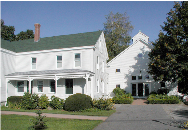
Photograph 3: Finished Roof Back Then – Looked pretty good seventeen years ago. New shingles were installed over a fully adhered membrane applied directly to the original roof decking.
