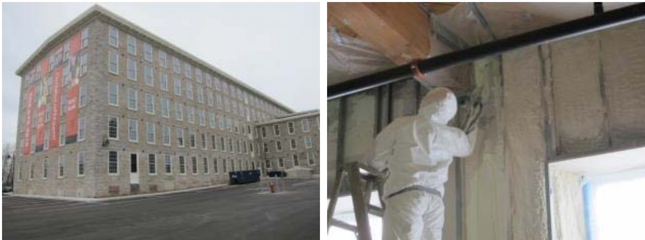
Figure 1. Mass masonry retrofit project overview (left); interior insulation at beam ends (right)
