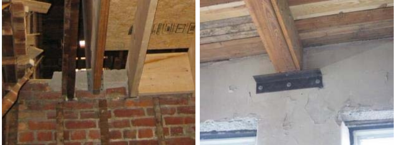
Figure 75. Transfer of load from masonry using joist hanger (left) or structural angle (right)
