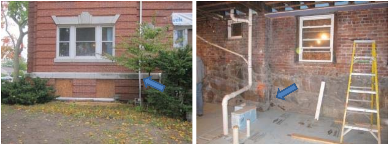
Figure 26. BSMT-W1 and BSMT-W2 joists showing water deposition at wall jog
