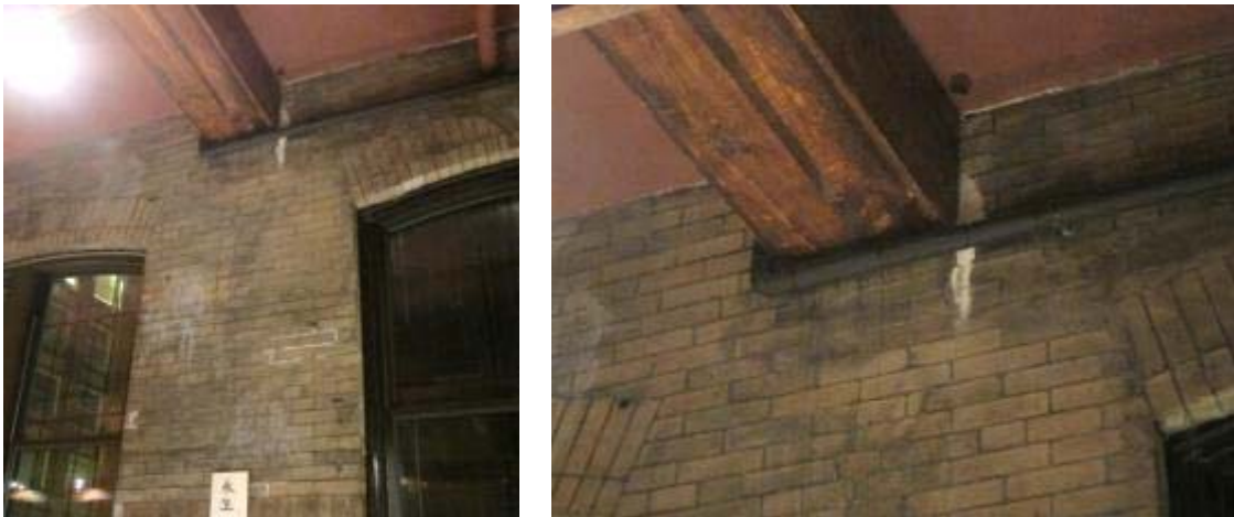
Figure 67. Evidence of water penetration at embedded beam end in masonry
