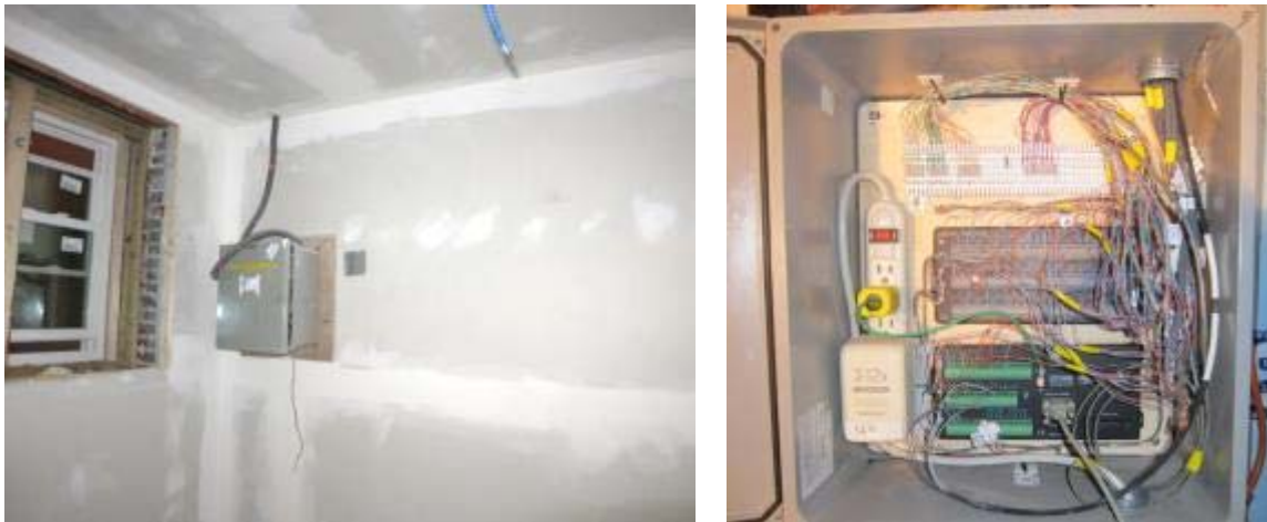
Figure 37. Data acquisition system showing placement (left) and wiring connections (right)
