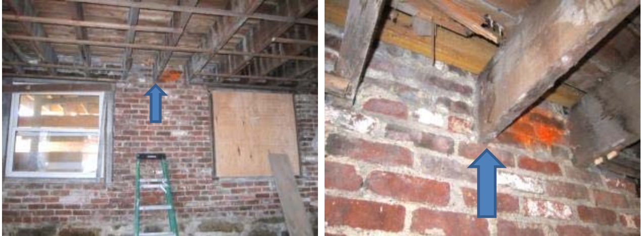
Figure 25. BSMT-E2 joist, showing existing water staining
