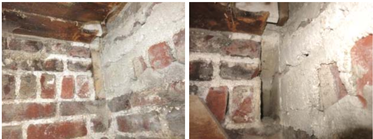
Figure 61. Joist end stub embedded in wall (left); joist pocket showing mortar (right)
