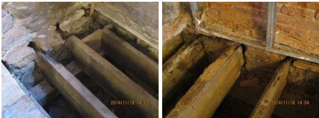
Figure 12. Damage to embedded beams at walls
