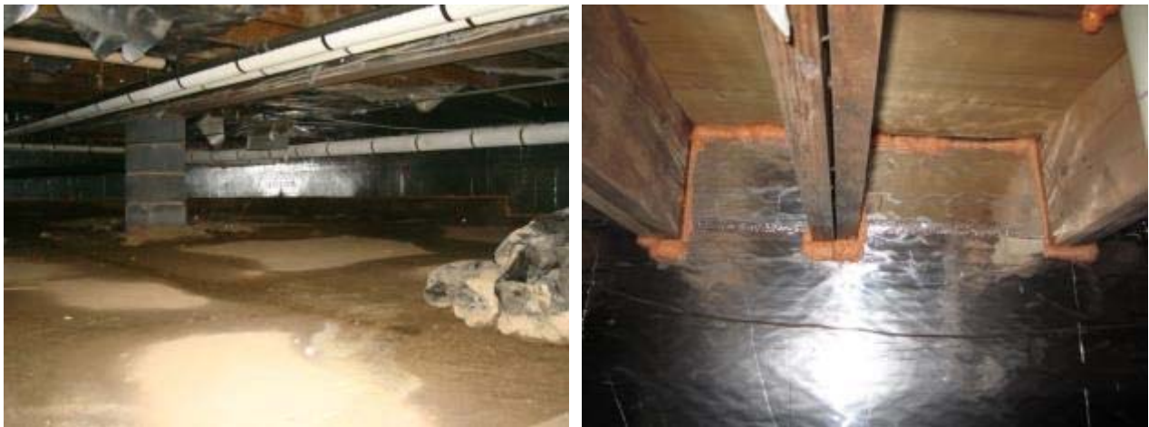
Figure 3. Postretrofit crawl space conditions (left); insulation board sealed at joist ends (right)
