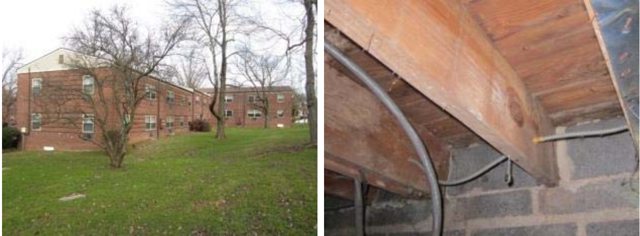
Figure 2. Overview of apartment complex (left); preretrofit joist ends in concrete masonry unit walls (right)
