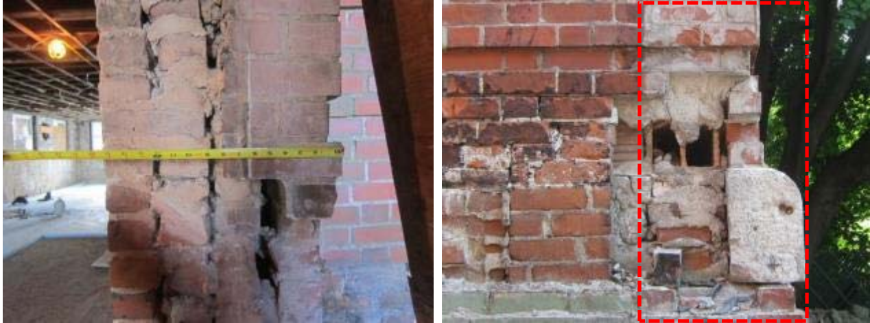
Figure 17. Wall section at solid brick (left); at hollow clay block infill (right) conditions
