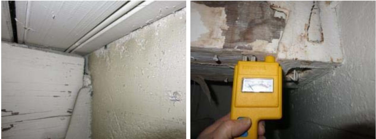
Figure 9. Wood clear of masonry (left); low MC despite wetting stains (right)
