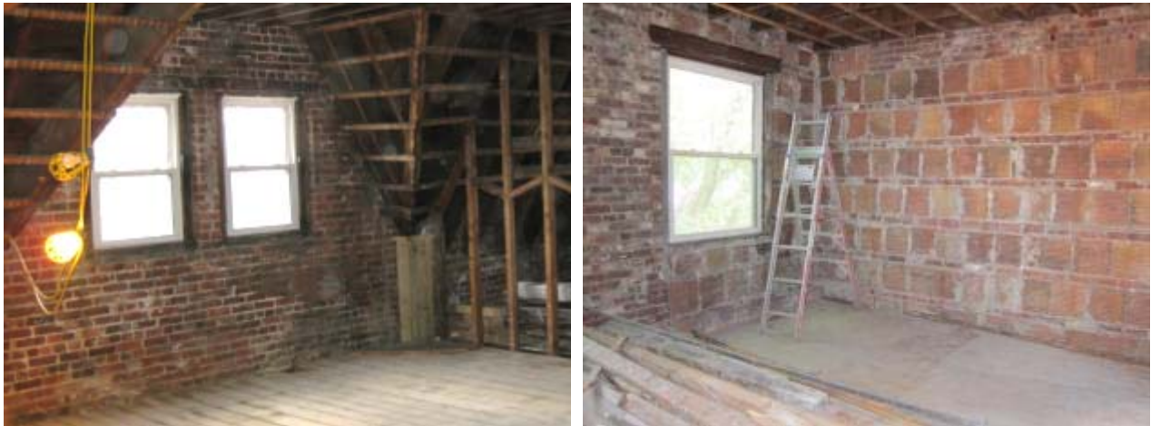
Figure 16. Exterior wall conditions at solid brick (left); hollow clay block infill (right)
