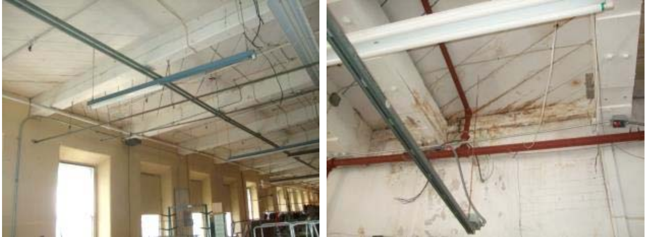
Figure 5. Typical large beam geometry (left); water damage at beam end (right)
