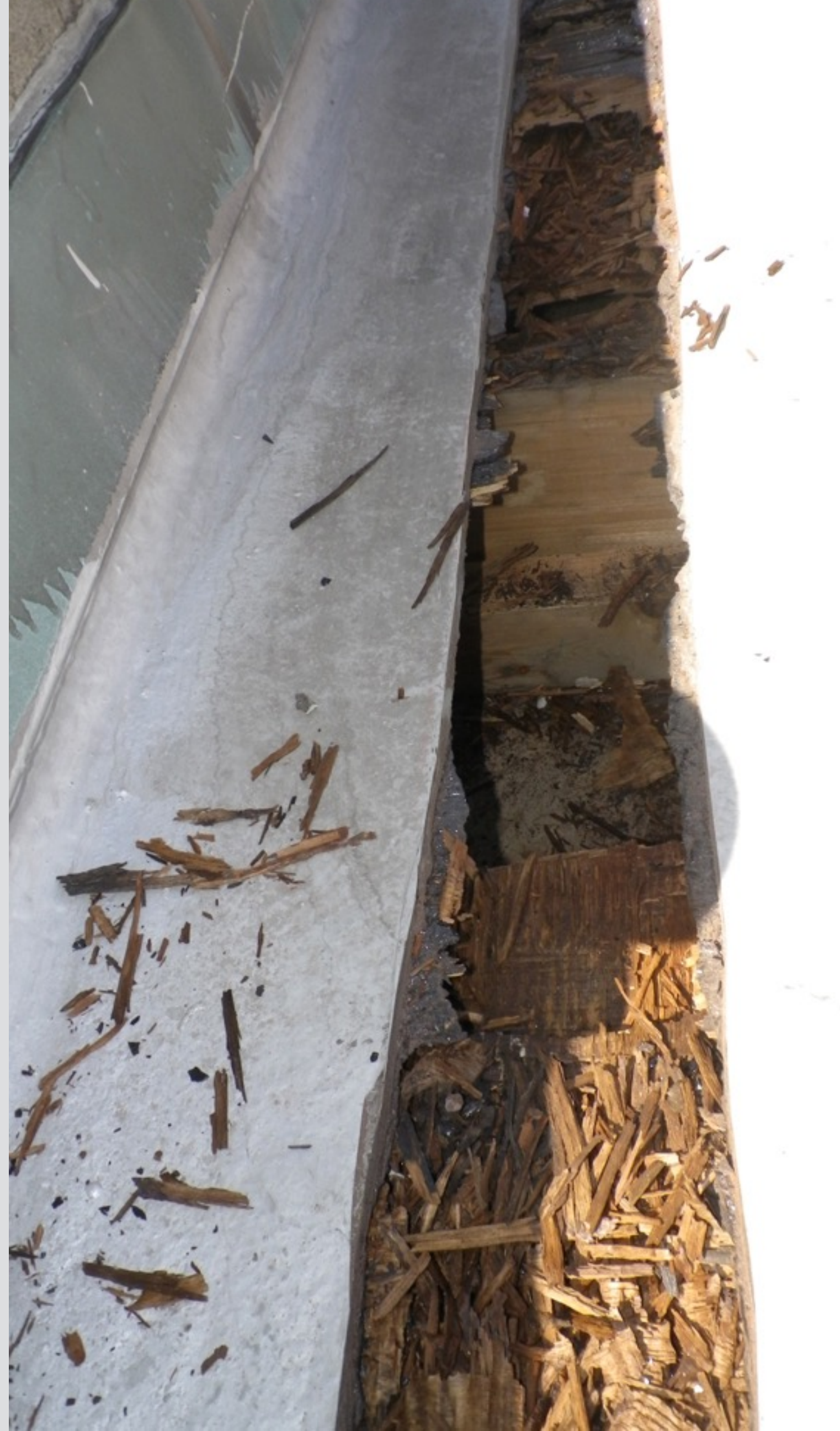
Water rotted out wood deck. Leak is not due to the membrane. Parapets and coping are to blame.
