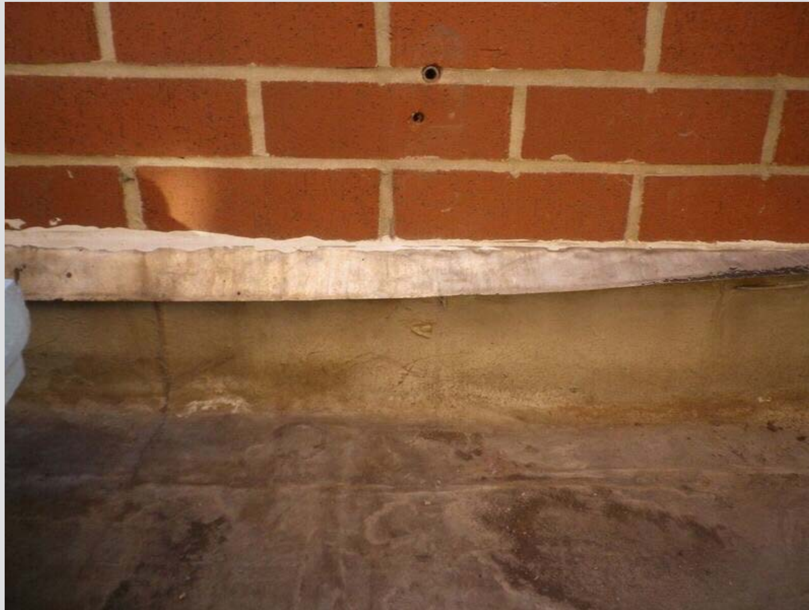
Cut-in base flashing. Face sealed. No possibility to drain out.
