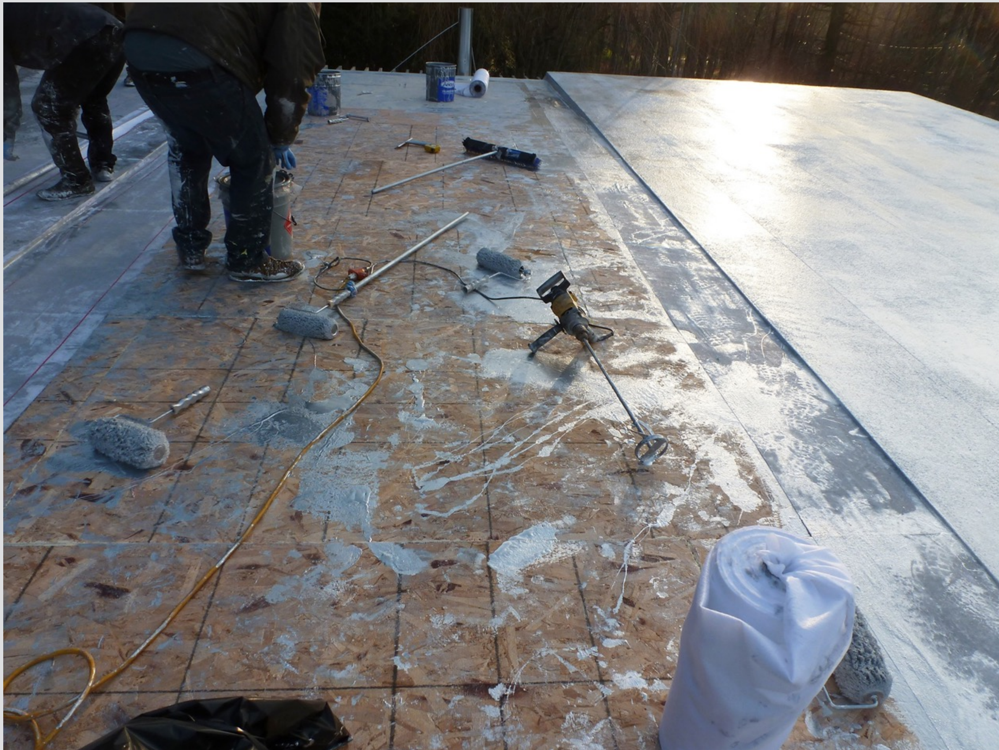
How do you ensure application thickness? Roof pitch \frac{1}{16} - \frac{1}{8} per foot
