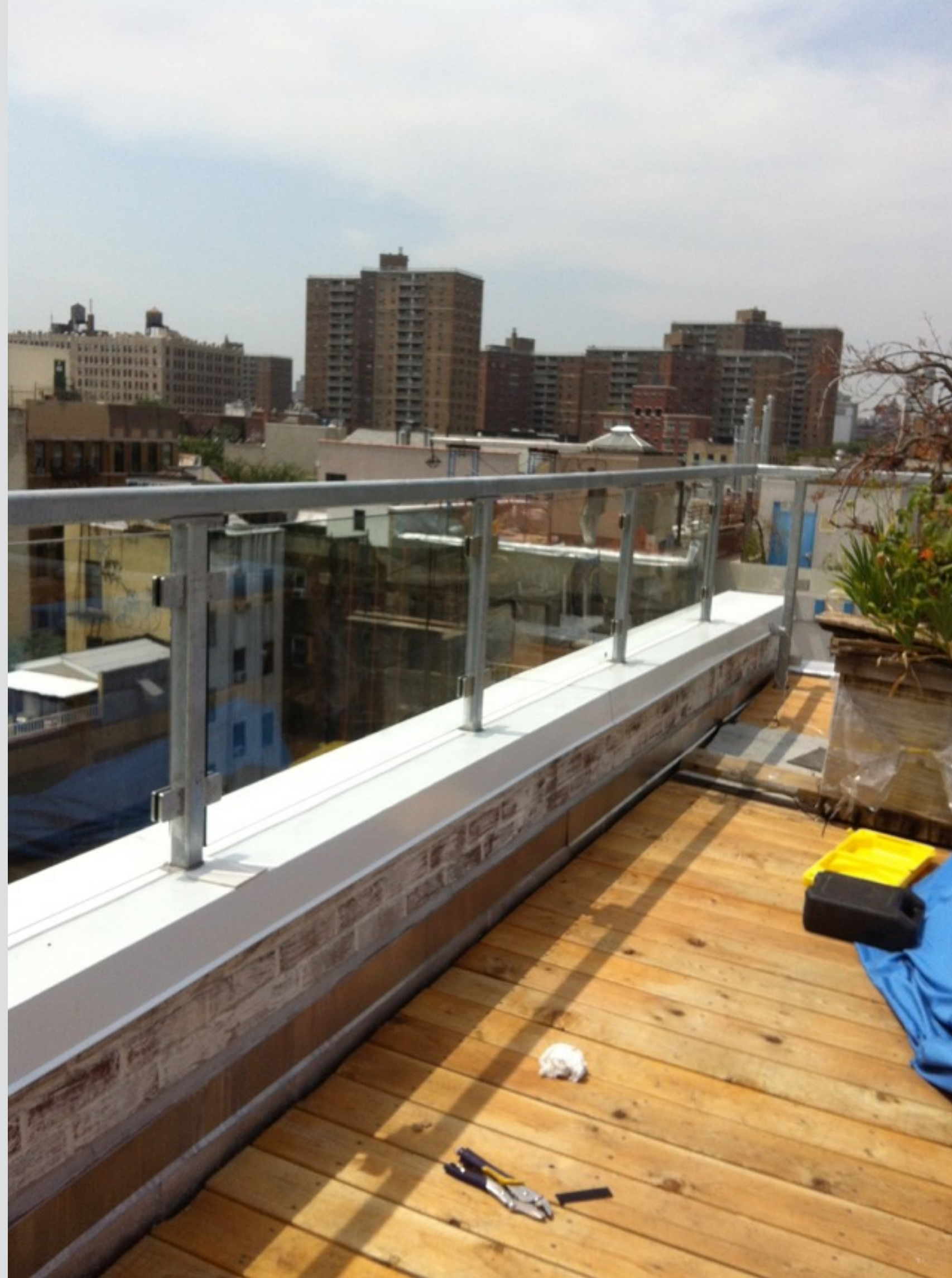
New and rebuilt masonry. Peel and stick. Aluminum cap, core drilled posts. All steel was prefabricated and then sent to galvanizer and bolted together on site.
