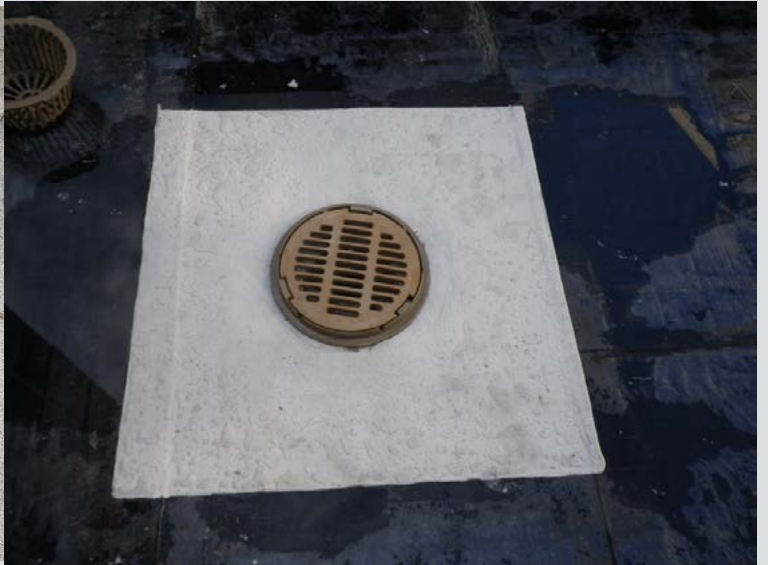
Cutting and patching membrane to get it into clamping ring at critical point of system
