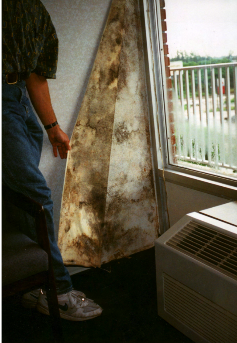
Photograph 1 Mold Contamination in Hotel Room
